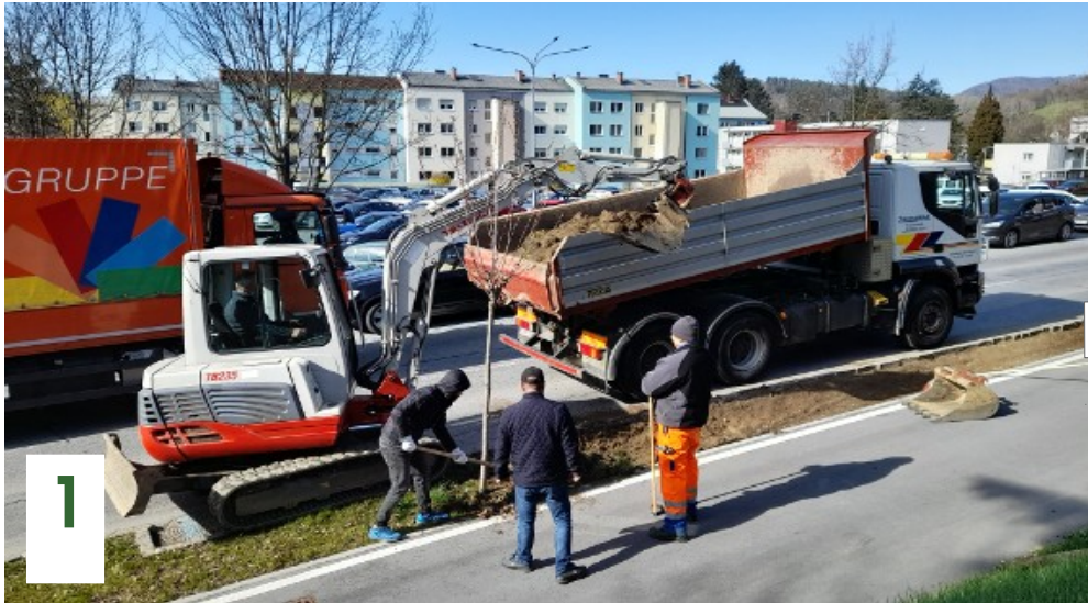
Removing vegetation and top soil, cleaning out roots of weeds by hand
